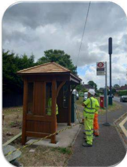
Replacement bus shelter on Fir Tree Road (A2022) with Sycamore Rise, Banstead, SM7
