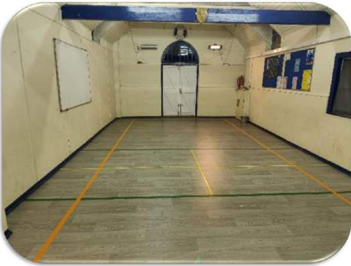
Figure 8: NW121 The repair of the sub-floor, and replacement of the floor surface (Phase 1 of Tadworth Scouts HQ's upgrade) at The Green Hall, Dorking Road, KT20 5SL.
